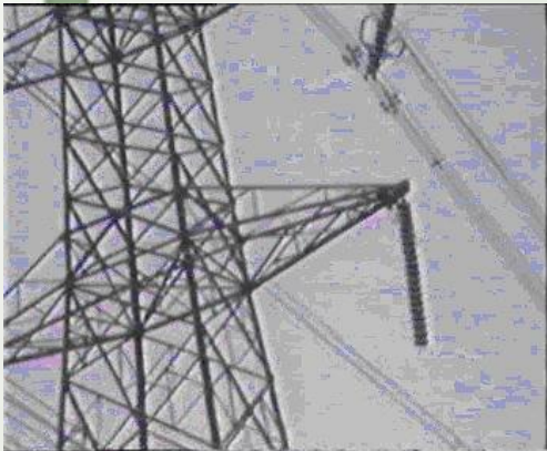
Insulator string broken during galloping
