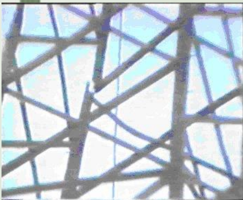
Tower member broken during galloping
