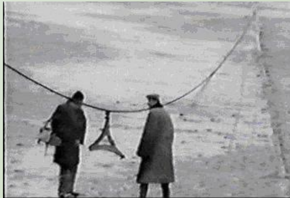
Spacer damper broken due to galloping
