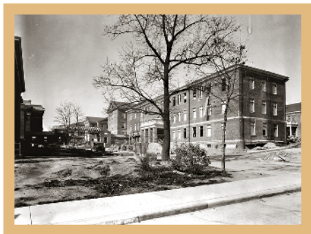
1929, Construction of new Isolation Ward; tree in left rear, behind truck, is Georgie Newport's Catalpa tree
