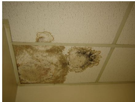
The stain indicates a leaking pipe in the ceiling. Such leaks can create the environment for growth of mold and mildew, some of which can be toxic.
