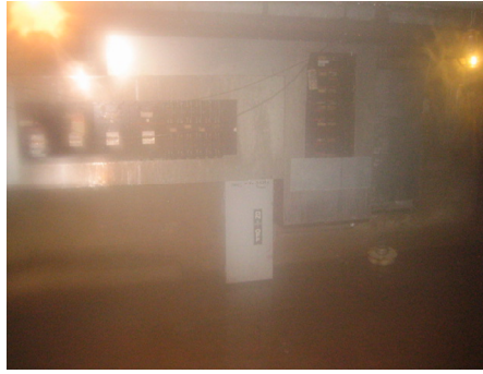
A steam leak in an electrical area could result in a power outage, along with other failures and damage.
