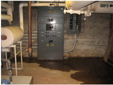
A water leak near a high voltage electrical panel has the potential to cause a deadly explosion.
