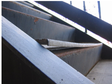
A stair tread in need of immediate repair. The unrepaired tread is a serious trip hazard on a busy stairwell.
