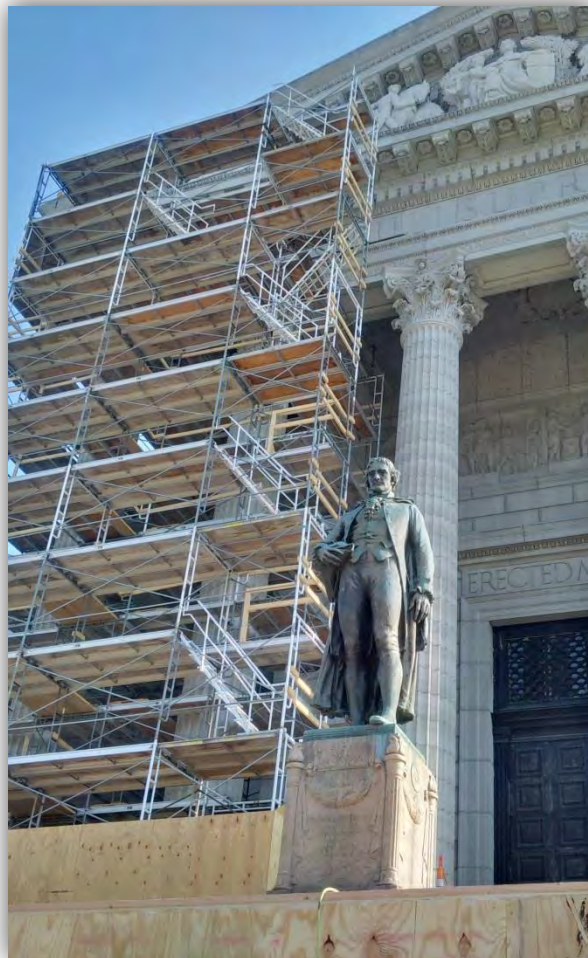
Scaffolding arises at the south entrance in preparation of assessment of the stone pediment - September 2015
