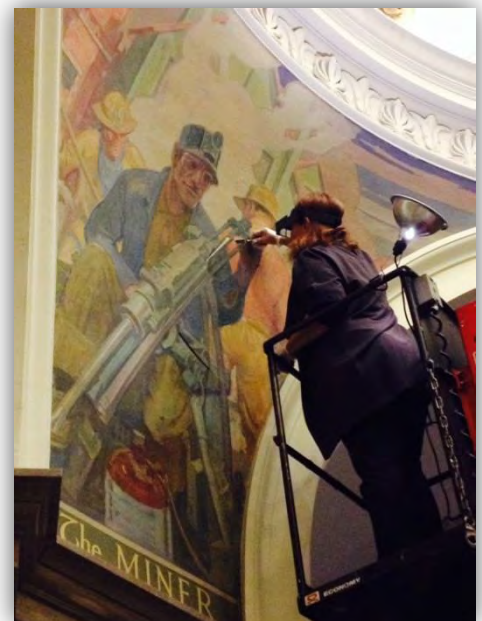
Peggy Van Witt of Van Witt Fine Art Consulting repairs a detached canvas panel on one of the Allen True "Occupation Murals" located in the Capitol rotunda.
