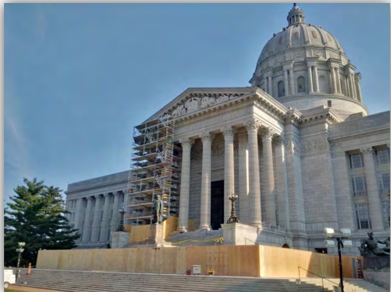
The south facade of the Capitol undergoing preparations for repairs to the facade and substructure.
