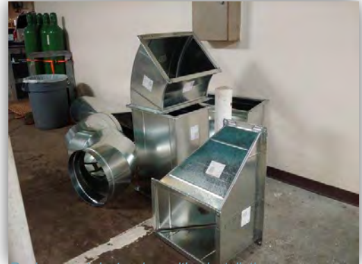
Replacement ductwork awaiting installation; one component of the first phase of the HVAC upgrade.
