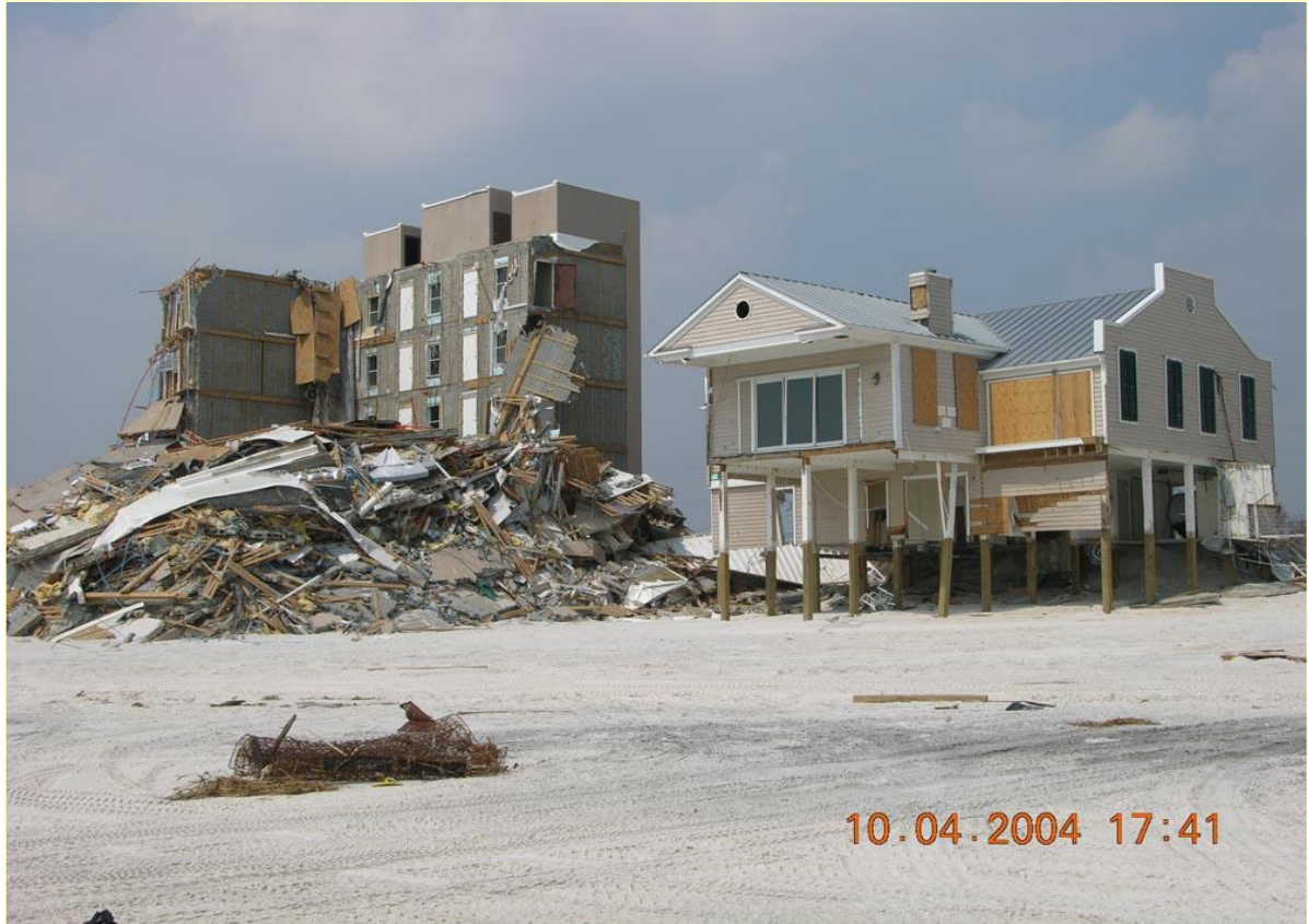
Figure 1. A five-story condominium in Orange Beach, Alabama, collapsed when the dune underlying its foundation was eroded during the September 2004 landfall of Hurricane Ivan.
