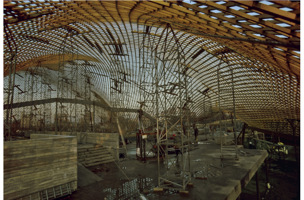
Figure 31: Mannheim gridshell 1974 by Mutschler & Partners, Freo Otto and Ove Arup & Partners - erection
