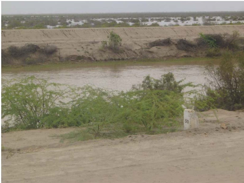
Plate 4: KPOD at RD 50 after receding of Water, Inundation Visible
