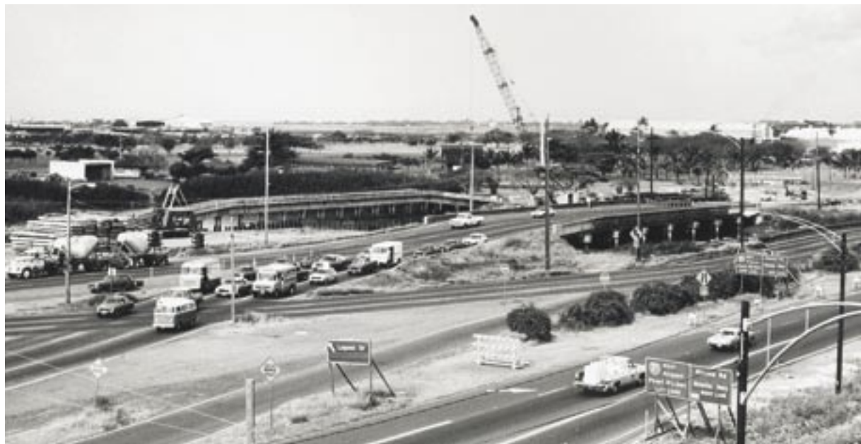
Above: Driving on Nimitz Highway in the vicinity of Lagoon Drive and Puuloa Road area was challenging during the construction of the H-1 Freeway.
