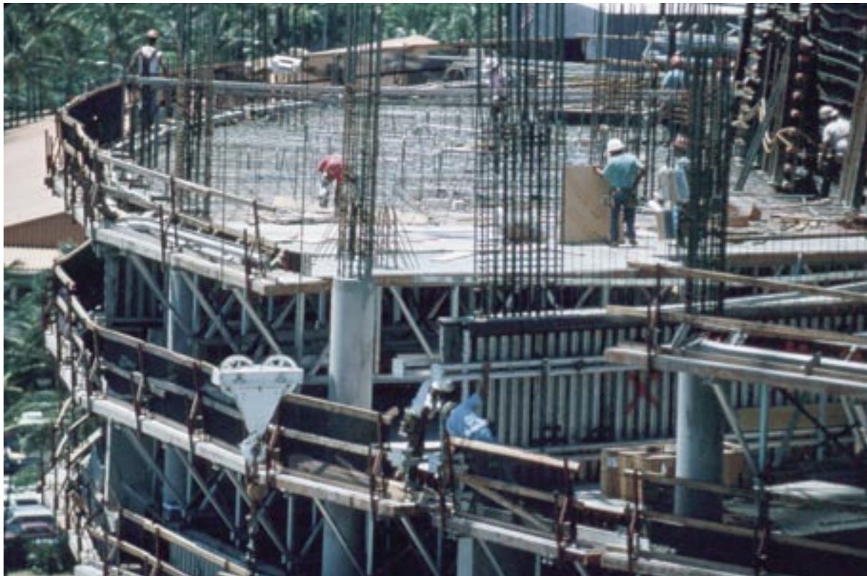
Below and opposite: Construction is in full swing on the seven-story Interisland Terminal.
