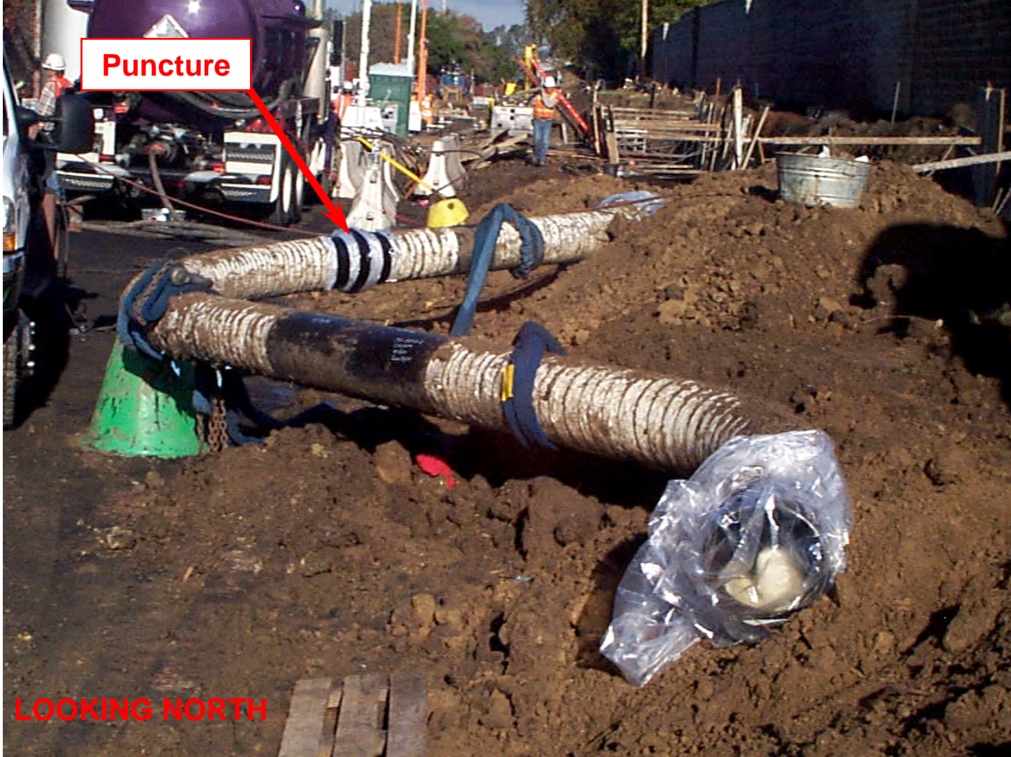
Photo Courtesy of CalOSHA
