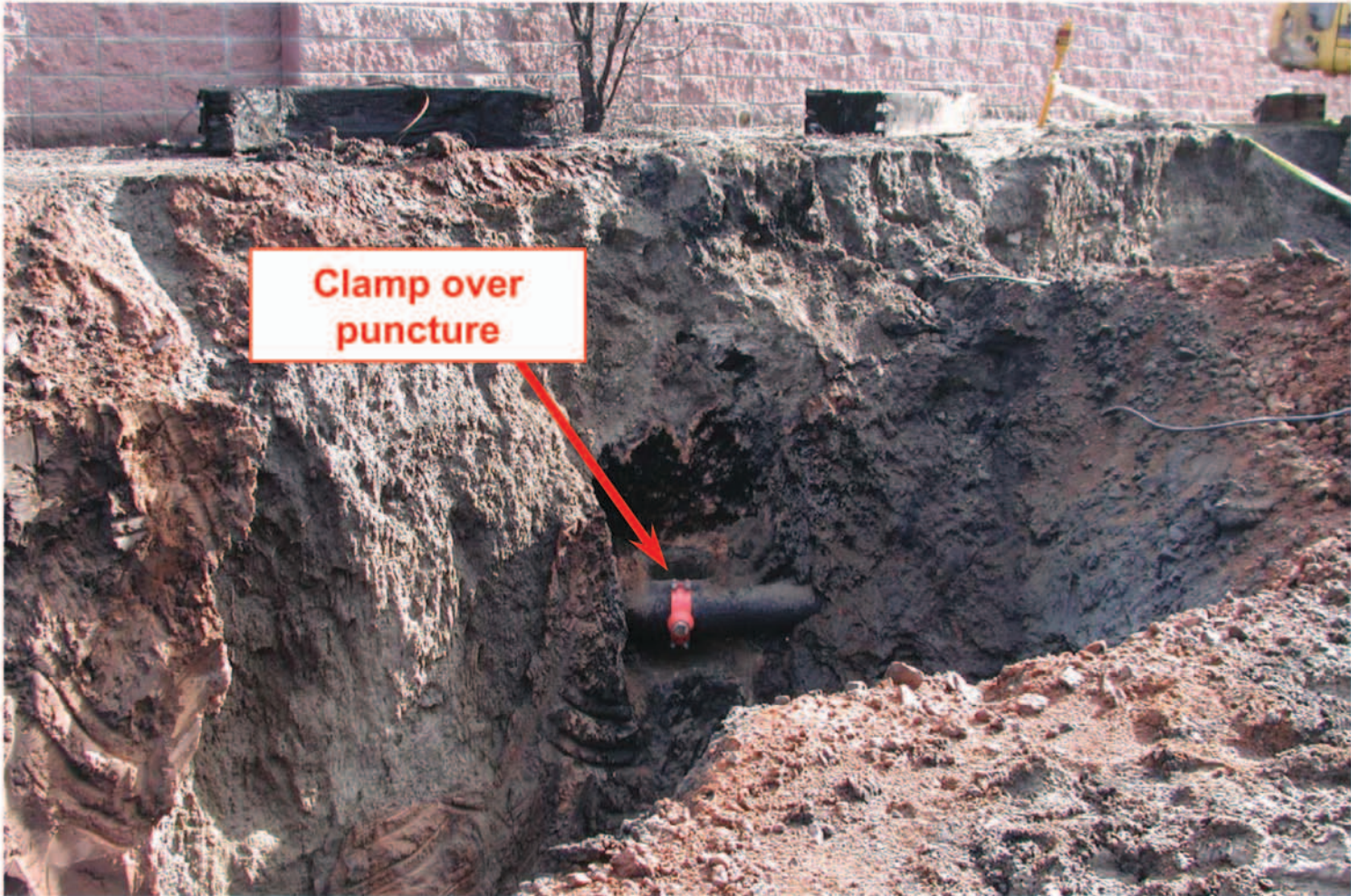
Photo Courtesy of CalOSHA
