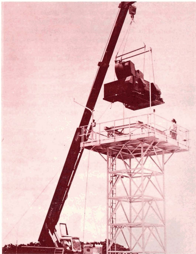
Improved Hawk radar is installed atop a 40-foot tower.
