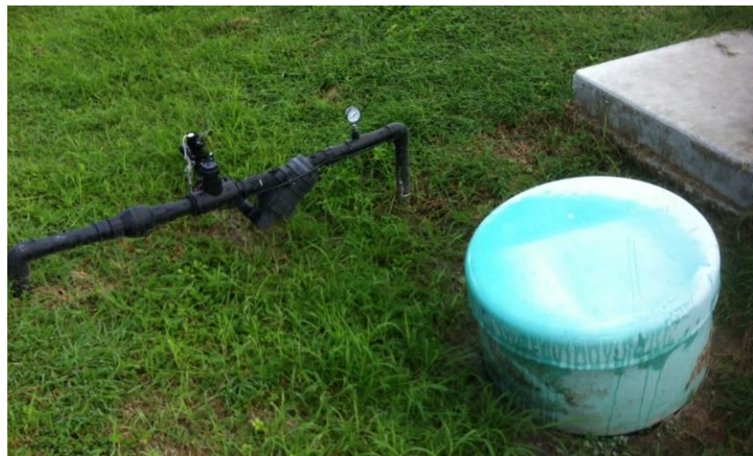
Figure 4-8. Rain Tanks© installed below a grassed bioswale at the RTPark 64 West Center are used to collect rainwater for non-potable reuse including irrigation, toilet flushing, and cooling tower recirculation.
