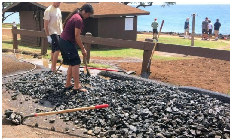
Bioretention design adaptations are based on underdrains and stone material: coral stone (top) and volcanic rock (bottom).
