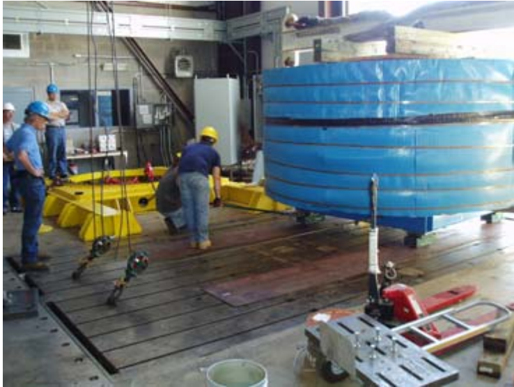
Figure 4-9. The generator was rolled into the dynamometer facility on a cart, which was pulled by cables connected to the gantry crane.
