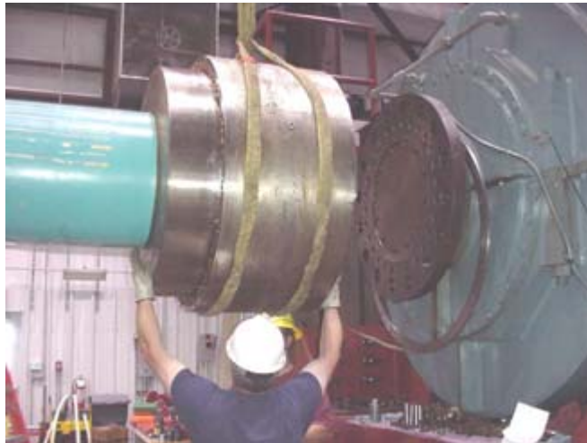
Figure 4-11. The coupling was installed after the generator and dynamometer shafts were aligned.
