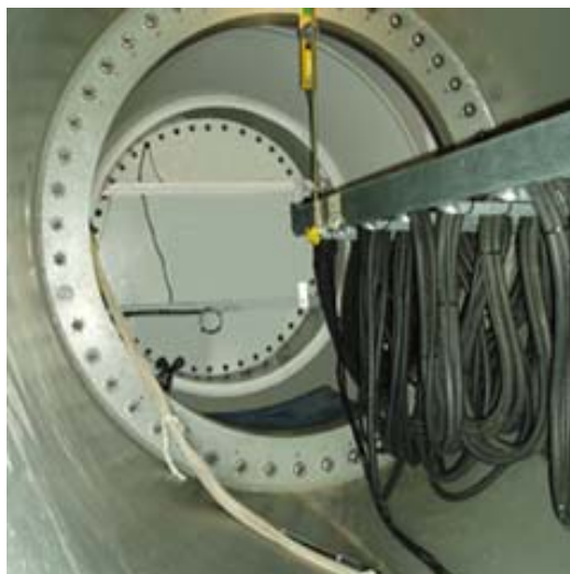
Figure 4-12. Droop loops were hung from the cable tray to take up the slack.
