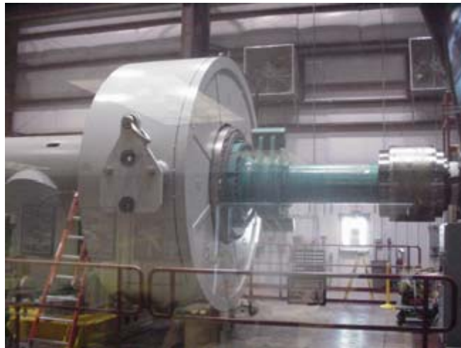
Figure 5-4. The generator connects to the dynamometer using a long shaft and coupling, as shown here viewed from the control room.
