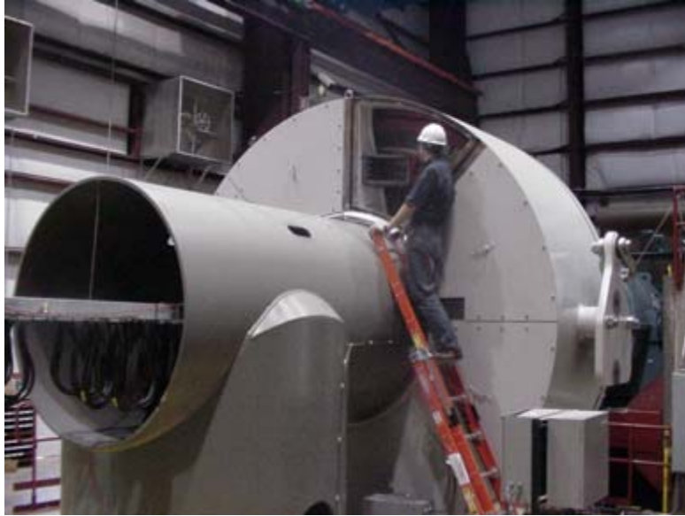
Figure 5-3. The generator was attached to the bedplate with a turret, and had removable covers for access to the active materials.
