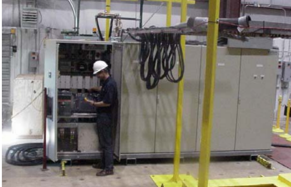
Figure 5-5. The power electronics connected to the generator via overhead trays, and connected to the grid via trays on the floor.
