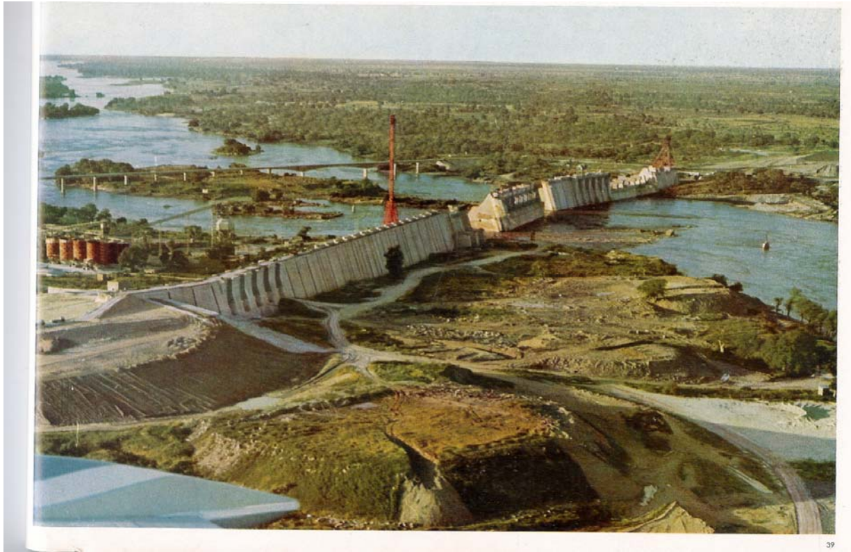
Fig 3.5: General view of the dam from upstream Photographs during construction of Roseries Dam
