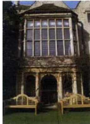
Fig. 7 The Doric order Loggia under the earlier cantilevered drawing room window (Reproduced with kind permission of McLaughlin Ross IIP Historic Building Report page 26)
