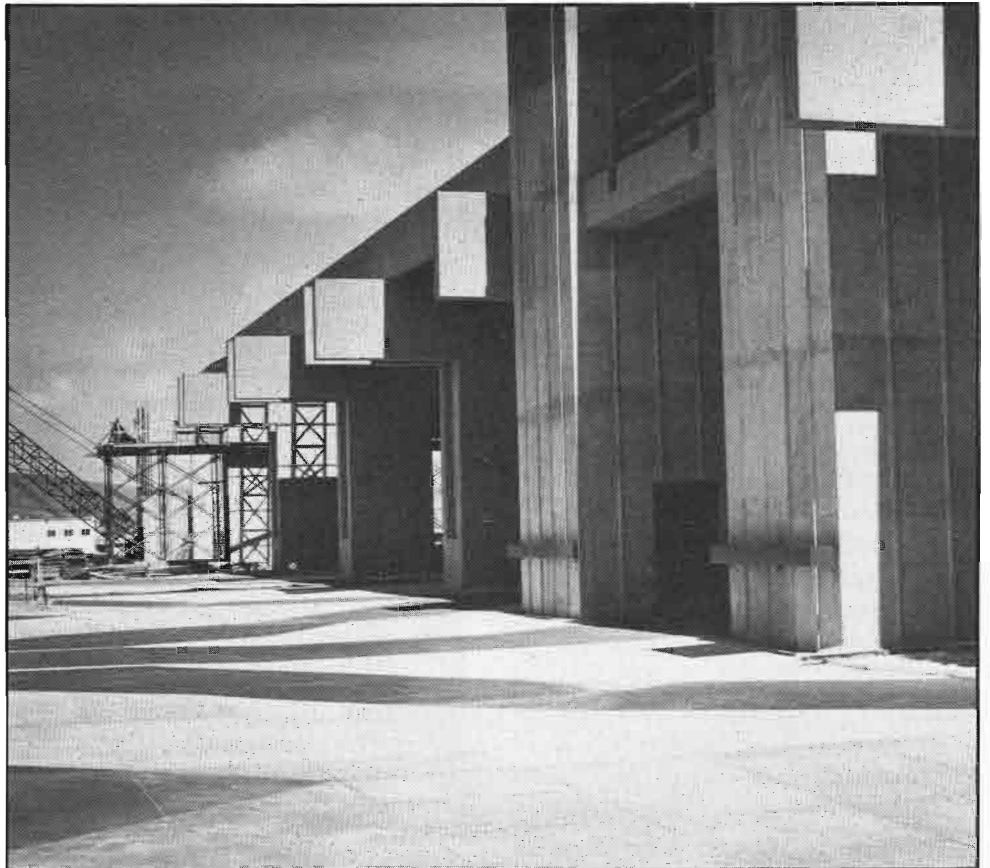
This 624 ft. extension at the Honolulu International Airport adds 19 new check-in counters and 10 new baggage claim devices.
