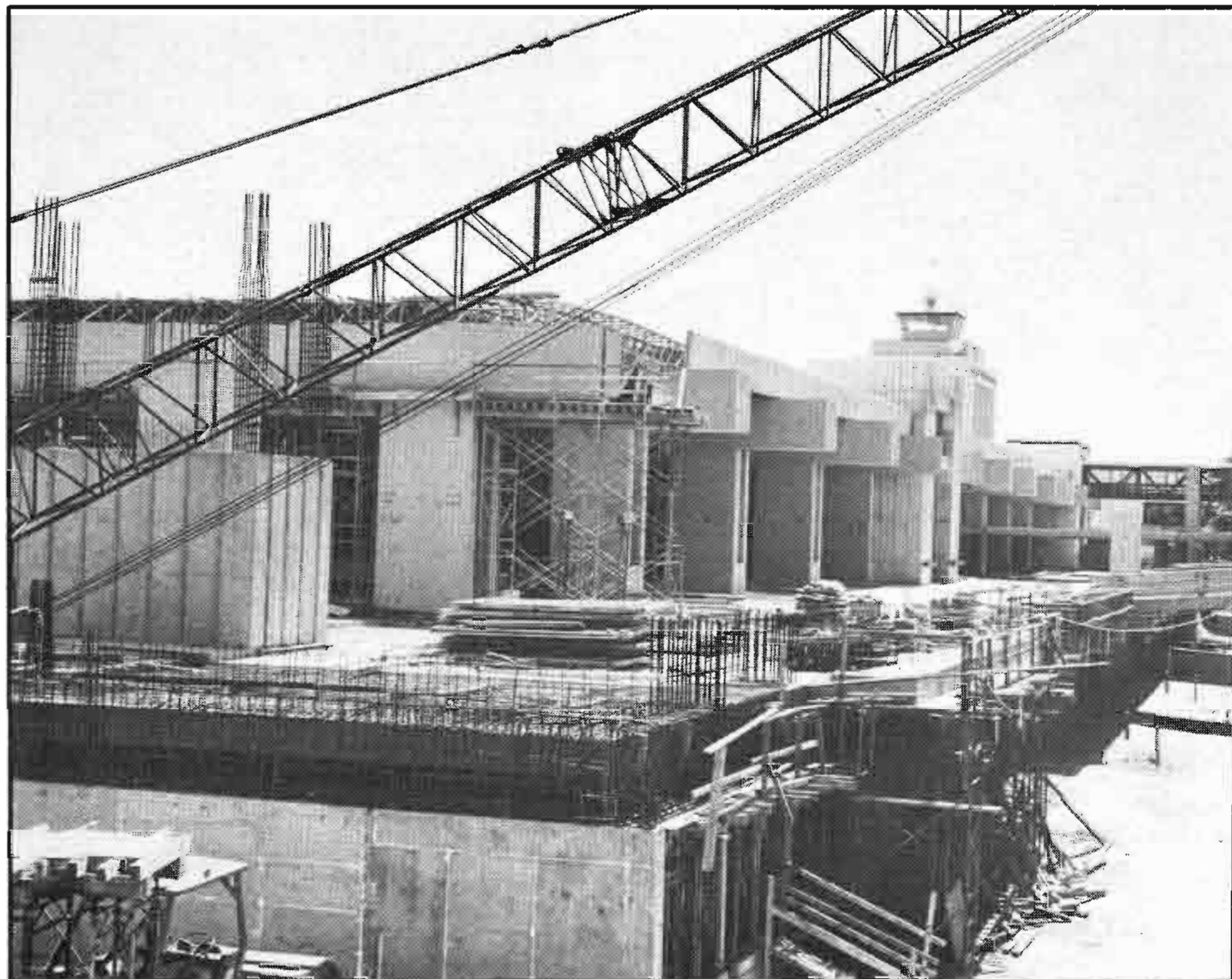
Construction continued on the Diamond Head Concourse of the Honolulu International Airport. Completion is expected in August, 1986.
