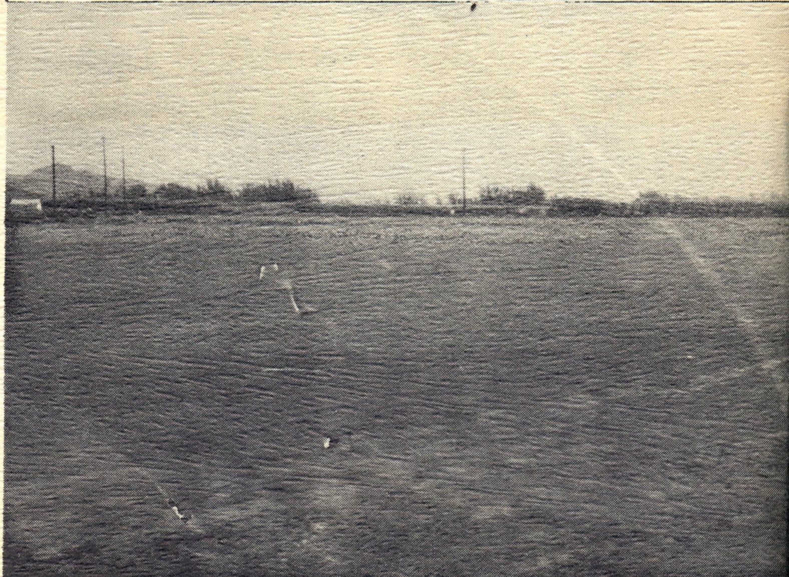
Pictures above show construction under way at the Lihue Airport. Top photo shows coarse rock ready for oiling on new taxiway. Picture below, finished grade, parking apron. Runway is completed. Passenger terminal building was completed in December, 1949. Other improvements planned include a freight terminal building and lighting system.
