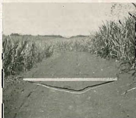
One of the contour drains in a soil erosion control experiment at Childers. This demonstration was put down by the Bureau.
