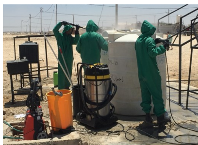
Disinfection of storage tanks in Za'atari @ 2016 UNICEF Jordan/Kamara
