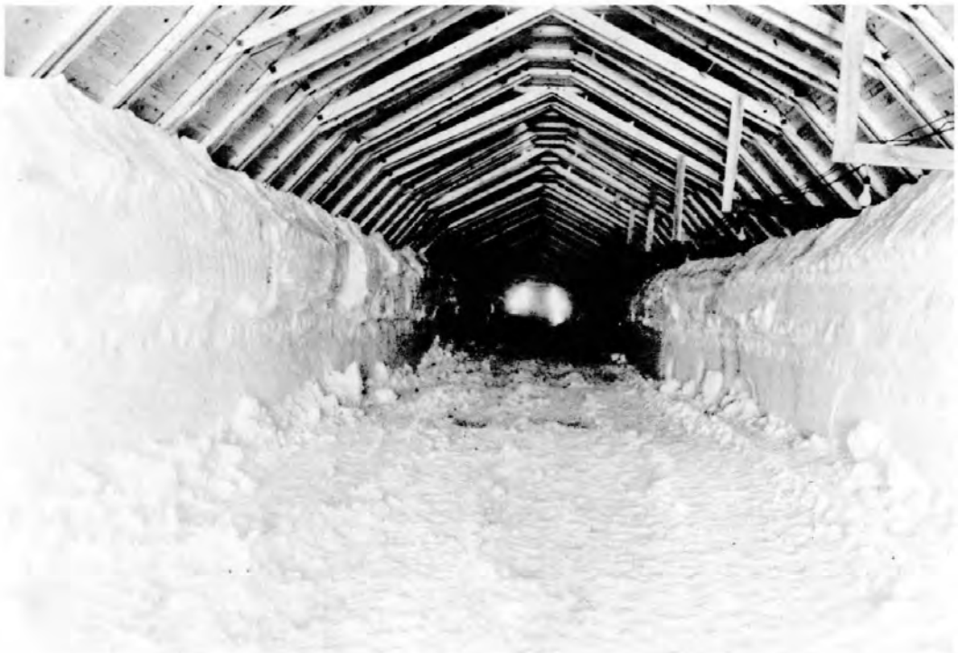
Figure 10. One of the open trenches covered with timber trusses. Photo taken before prefabricated buildings were installed.
