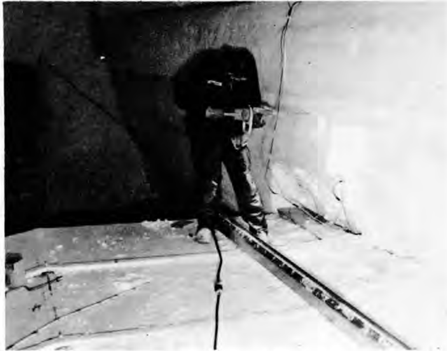
Figure 33. View from top of one of the T-5 buildings in a standard trench, showing a soldier using an electric chain saw to trim snow away from the building eave.
