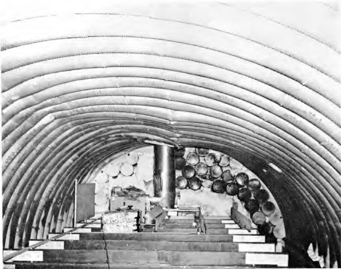
Figure 31. Deformation of Wonder Arch over one of the PM-2A buildings.
