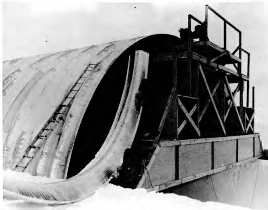
Figure 24. Wonder Arches being installed over 40-foot wide reactor trench at Camp Century.
