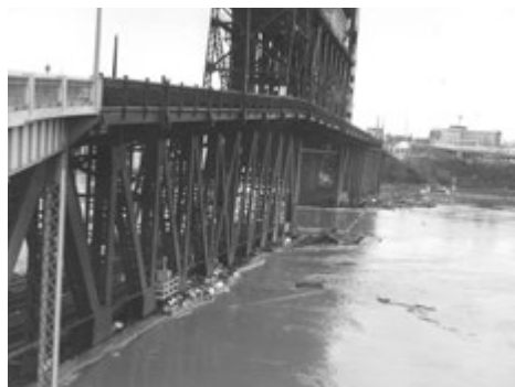
The lift span on Portland's Steel Bridge remains open to allow logs and debris to pass, taking pressure off the structure on Christmas Day, 1964.
