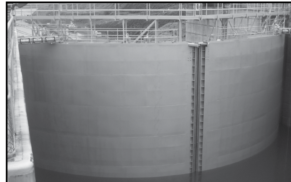
Jordan Reimer and Matt Hanson, Portland District structural engineers, and other TCX staff designed The Dalles’ 113-foot tall navigation lift gate with its 1¼-inch thick curved skin plate to meet current fracture and fatigue guidance. The team monitored all stages of gate replacement for quality assurance, from construction through installation.
