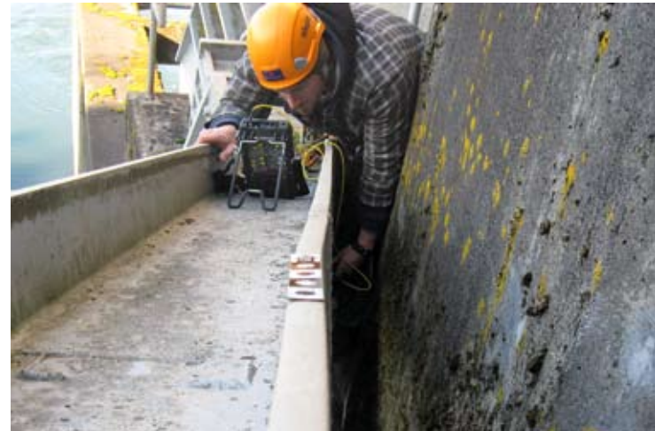
Inspections of many Willamette Valley dams’ spillway gates in the past few years found twisted, bent and buckled gate arms and structural members; cracks at structural connections; corroded wire ropes and connections; and other signs of stress.
