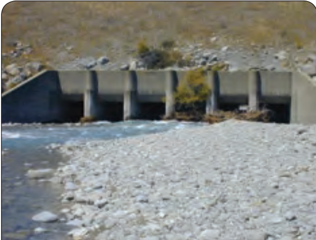
FIGURE 37 // Build up of debris upstream of Fork Stream culvert.
