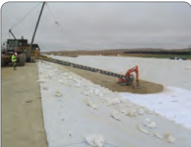
FIGURE 19 // The 'juggernaut' in action, conveying rock ballast material to the bottom of the canal.
