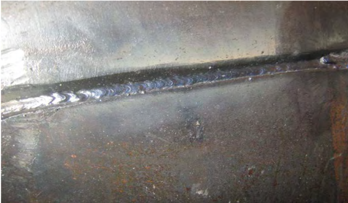
Root pass of a full penetration groove weld free of slag and ready for additional passes.
