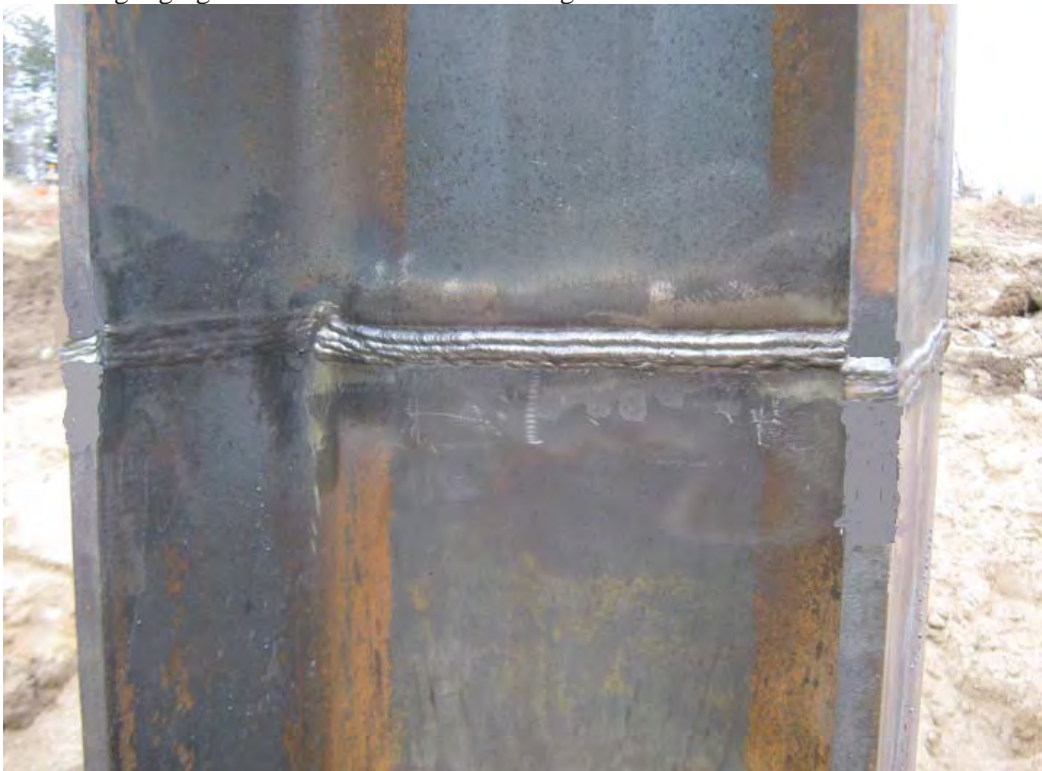
Completed full penetration groove weld. Note that all slag and arc strikes have been removed. Grinding and additional weld metal was added on the flange edges to correct minor misalignment.
