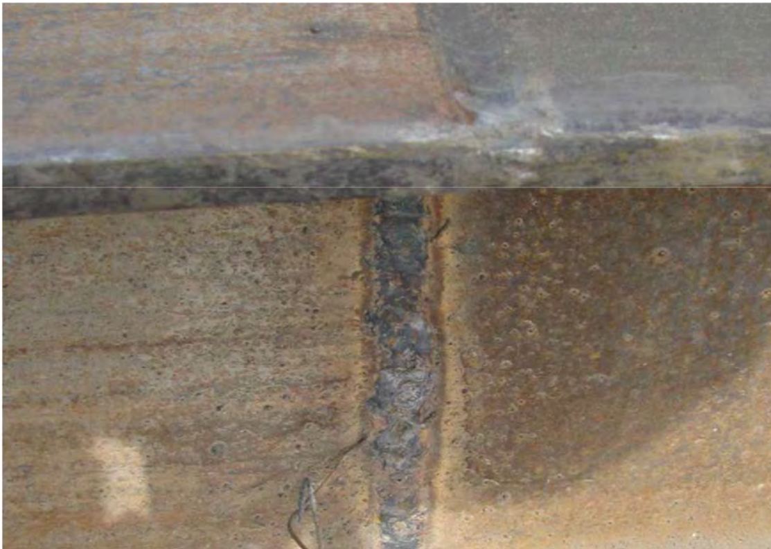
Under fill, use of an unapproved wire fed process (GMAW) - note wire protruding from weld.
