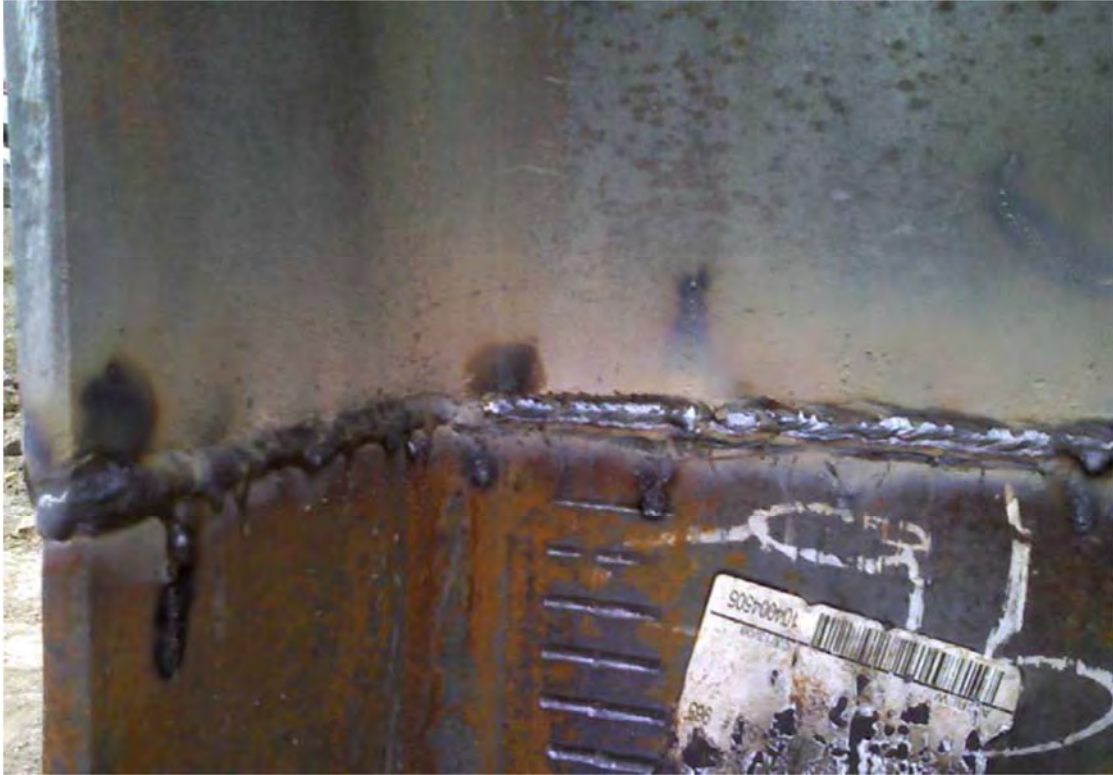
Slag, undercut, under fill, arc strikes.
