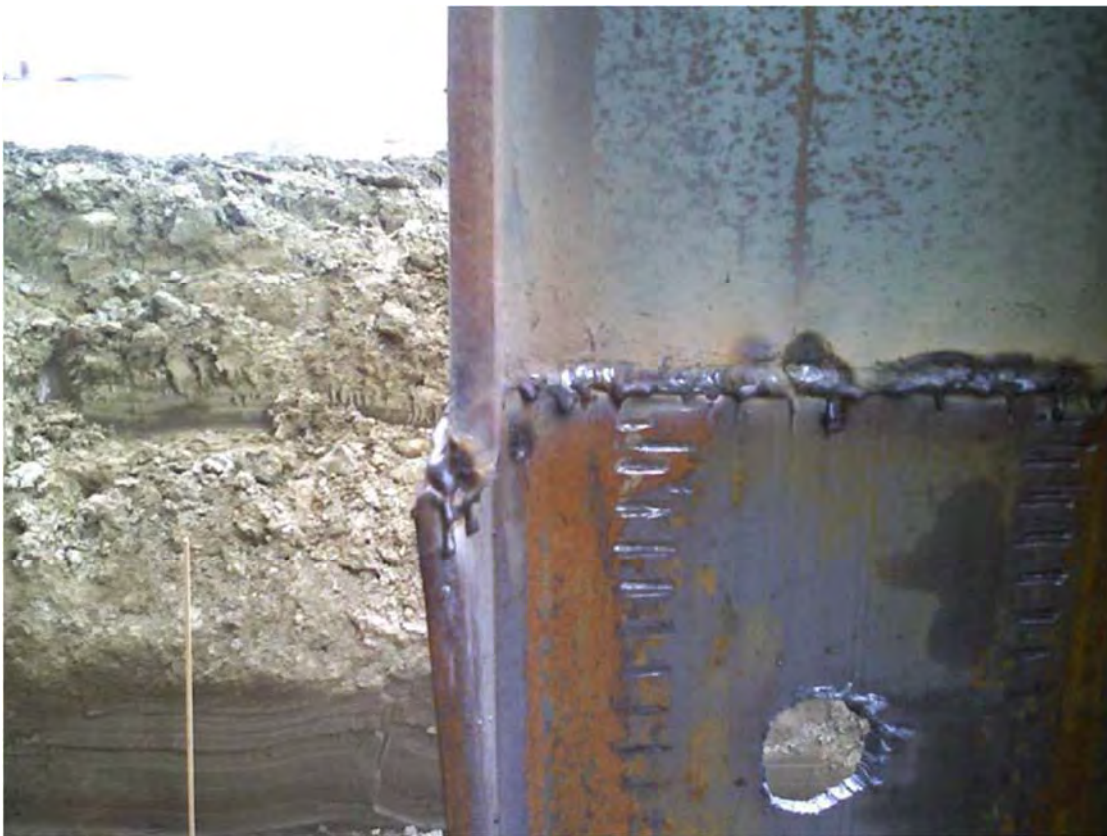
Misalignment, unacceptable profile, slag.
