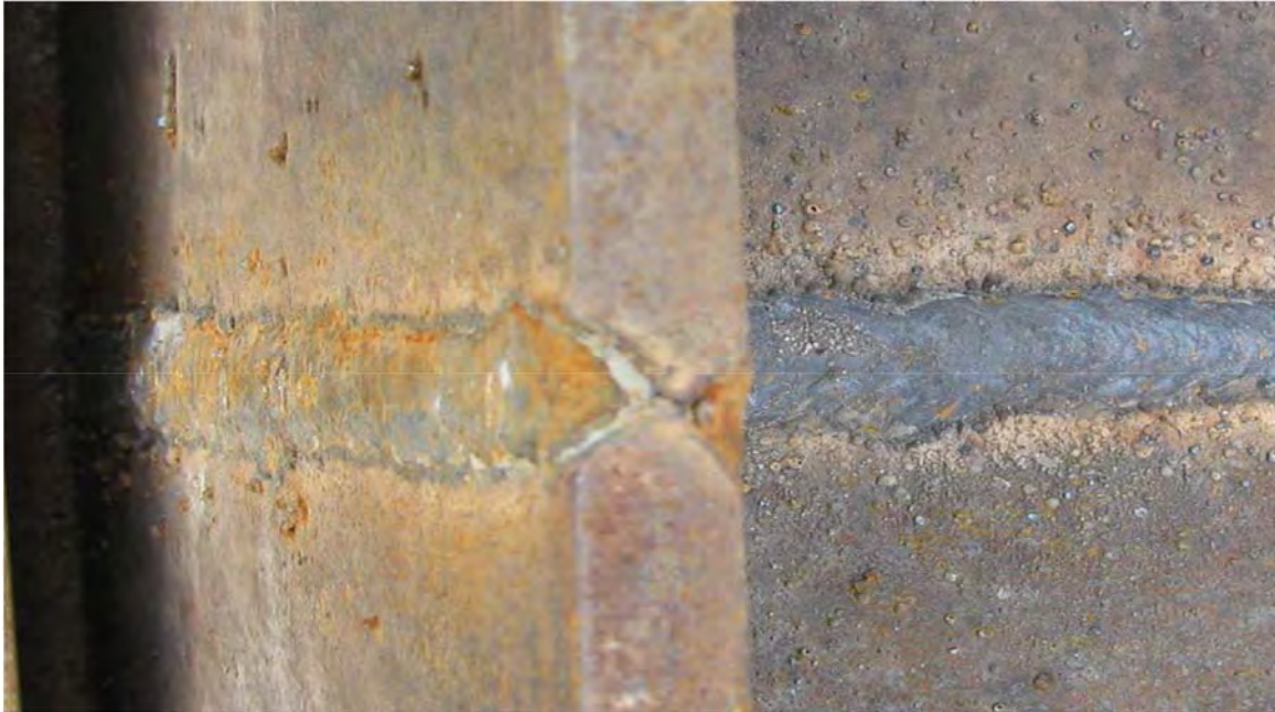
Insufficient back gouging and incomplete penetration.
