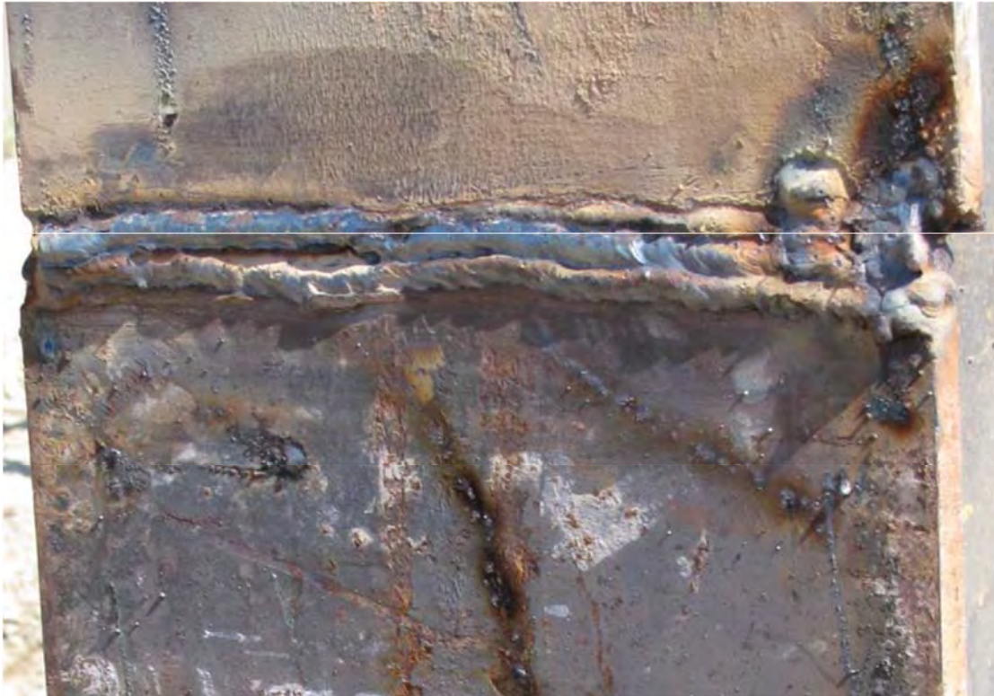
Misalignment, arc-strikes, unacceptable profile, contaminated surfaces, slag, undercut, porosity.
