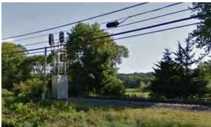
Exhibit 80: CTC Signal Mast on New England Central Railroad near Windsor
