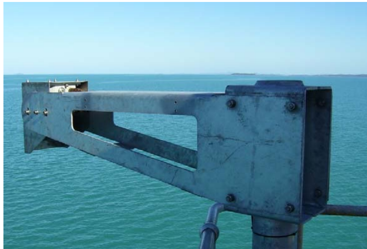
Figure 5 - Laser wave ranging gauge in operation at Hay Point.
