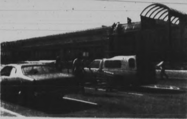
FINISHING TOUCHES — Workmen putting finishing touches on the exterior of the expanded ShopRite of Freehold supermarket.
