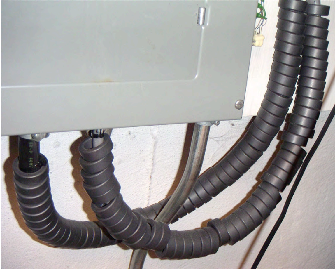
Figure 14: Common-mode chokes formed by stringing ferrite toroids like beads on two 3-conductor, 240-VAC power cables, one 60-A and one 40-A.
