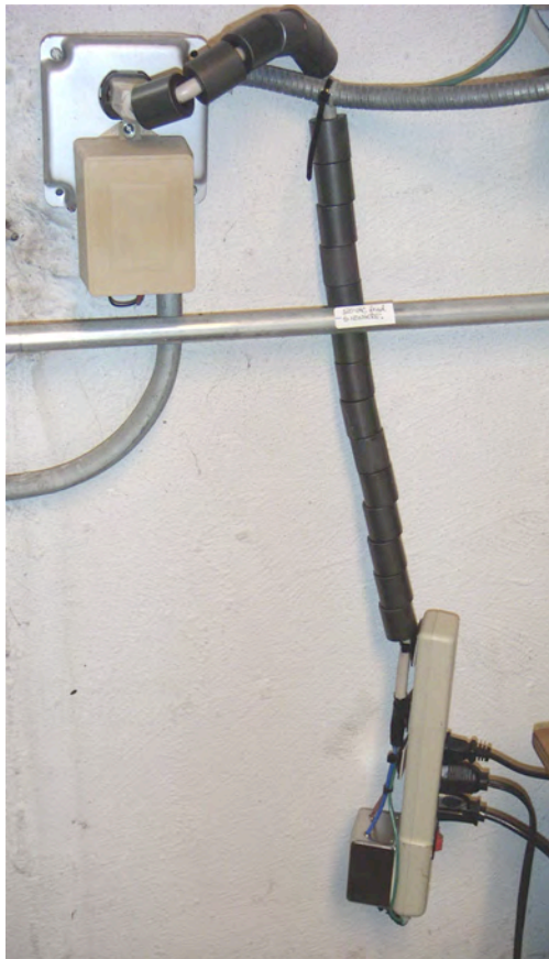
Figure 11: 15-A, 120-VAC, multiple-outlet strip with Corcom two-stage, L-C, difference-mode EMI filter and ferrite-bead common-mode choke added.
