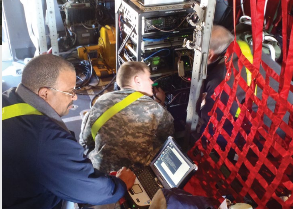
ARL engineers working with a Soldier while installing the system on an aircraft.
