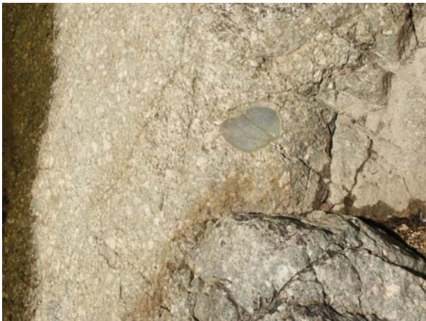
Fig. 17: Vaca Falls Dam Site - Granite Detail of the rock in the dam foundation area showing the massive nature of the intrusive macro-crystalline granite with its inclusions of sedimentary material.
