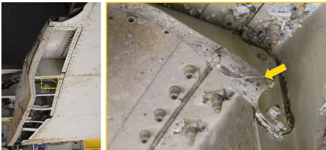
Figure 18: Outboard flap, damaged stiffeners within the seal pan cavity
