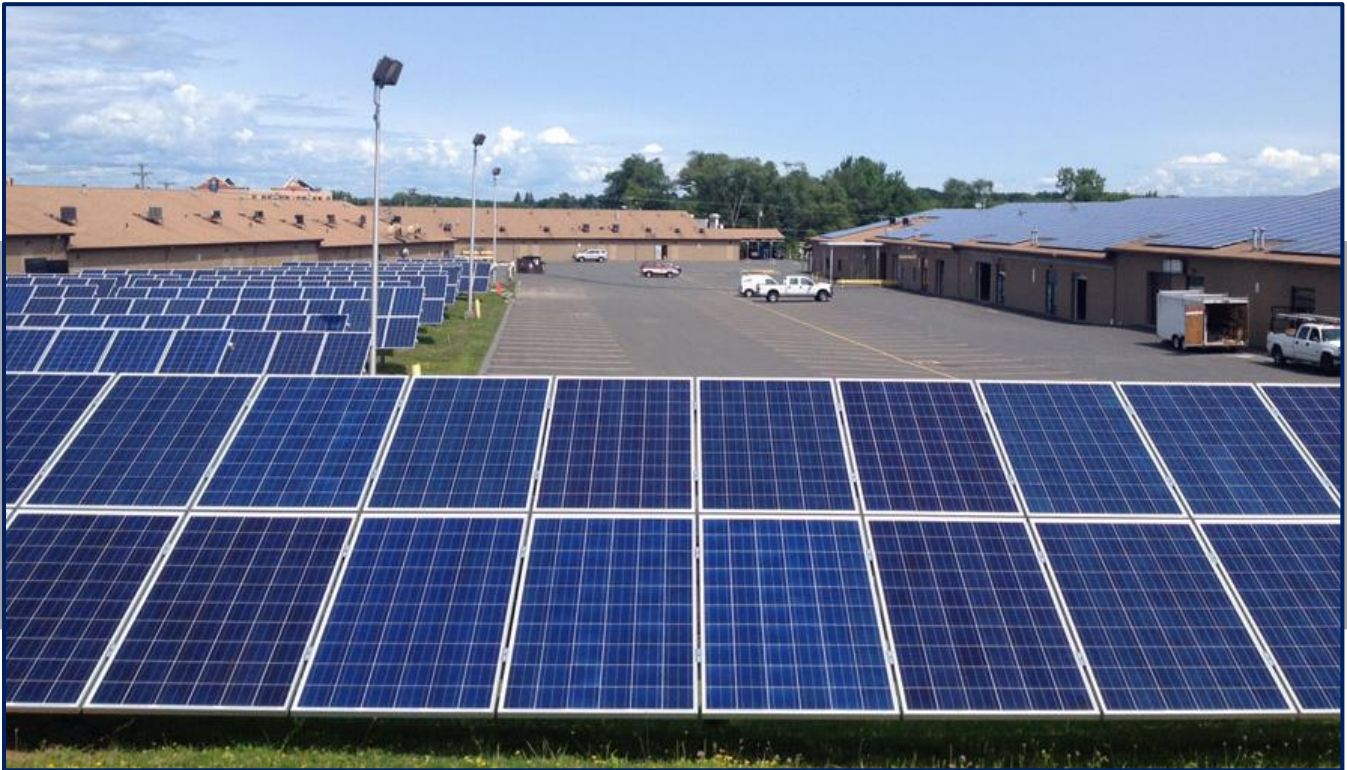
The solar PV system at Sofia's Plaza. Photo Credit: Connecticut Green Bank
