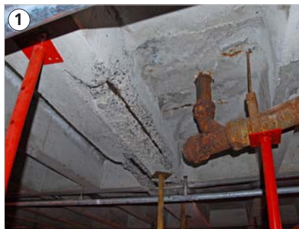
Infrastructure failure exemplified by the Substructure damage
