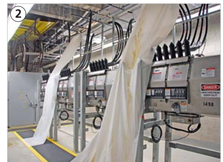
Water hazard on electrical equipment in Power Plant
