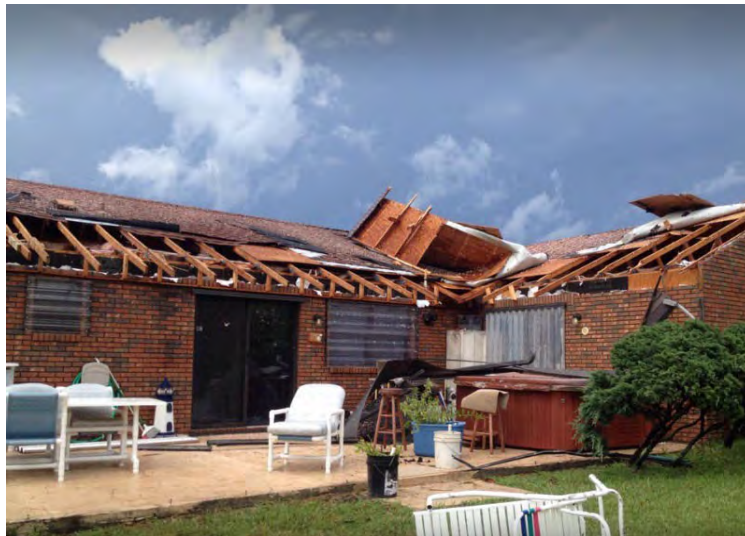
A picture of a large patio enclosure that was totally lifted from the concrete patio slab in Brevard County, Florida on September 13th, 2016. The patio enclosure was securely anchored to concrete and home with numerous 3 inch screws. Several large pieces of the metal patio were carried and deposited over 100 yards downstream, toward the northwest direction. Photo courtesy of NWS.
