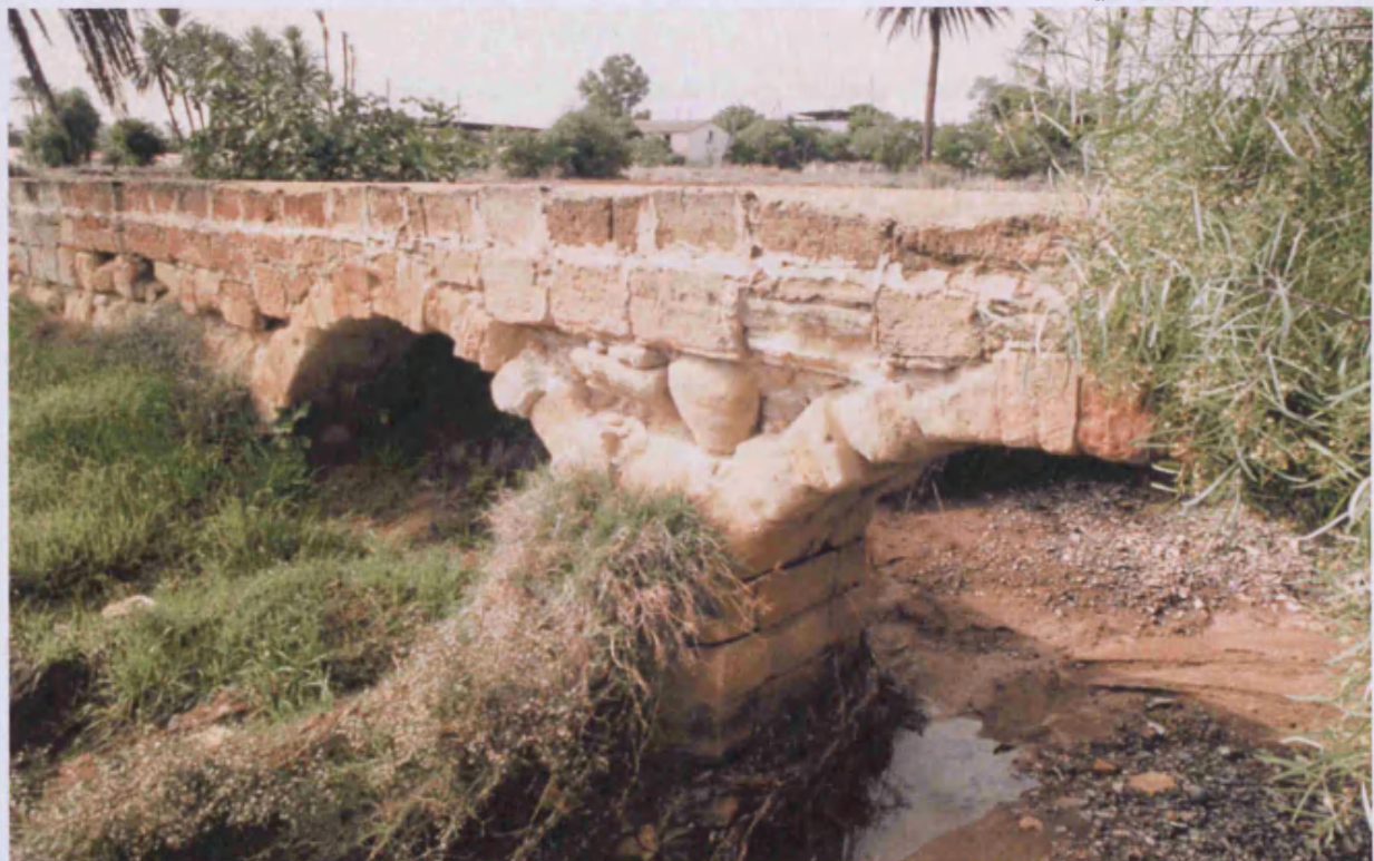
Part of aqueduct that may have provided the water supply to La Cava from the Nicosia area.
