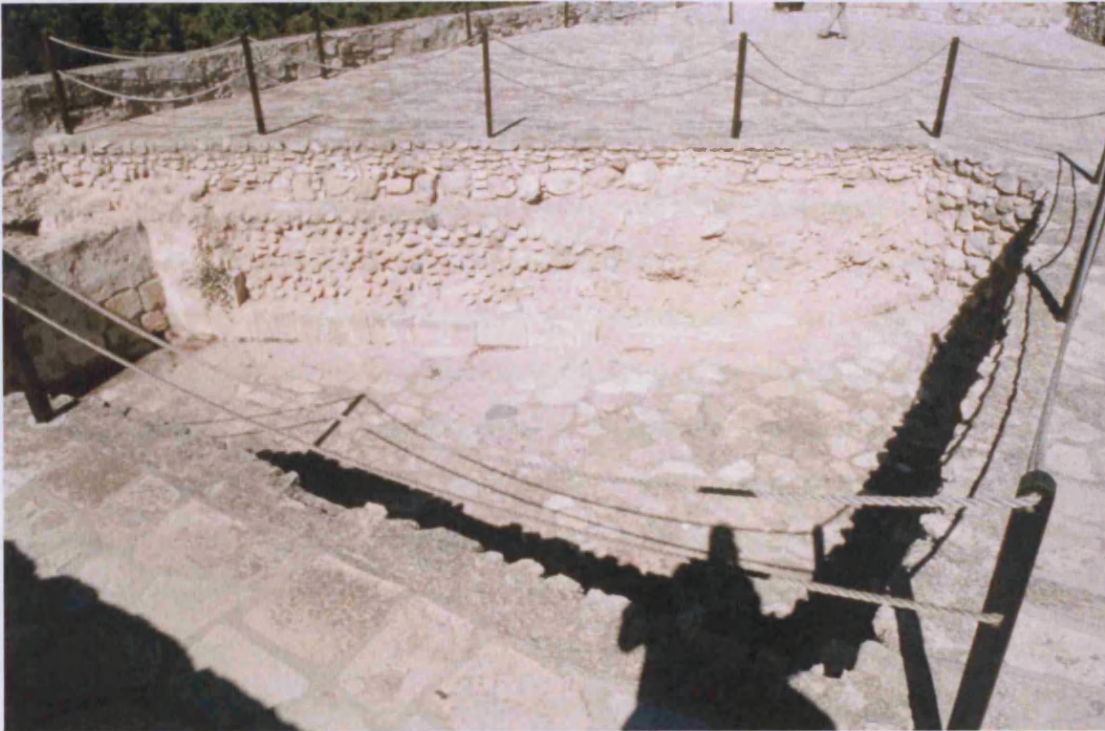
Uppermost level of the medieval pentagonal work, protruding above the surface of the later artillery platform.
