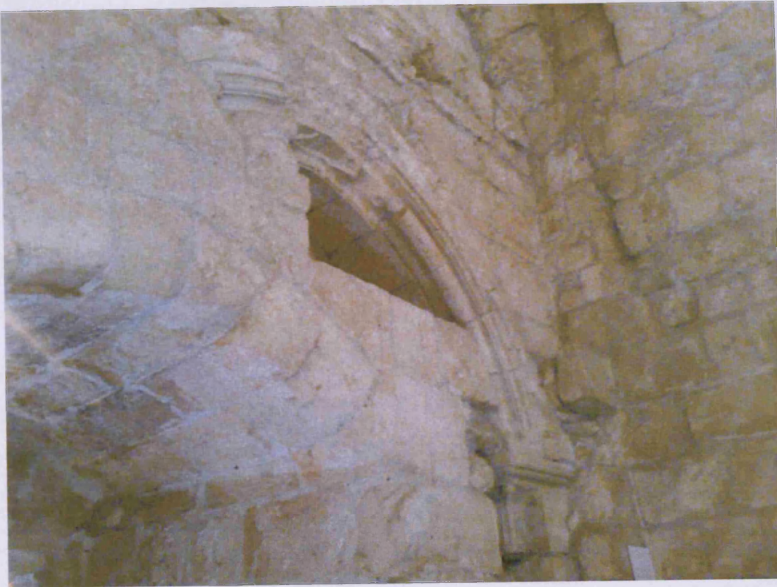
Partially blocked in pointed arch (4 on plan) within present entrance to the castle.
