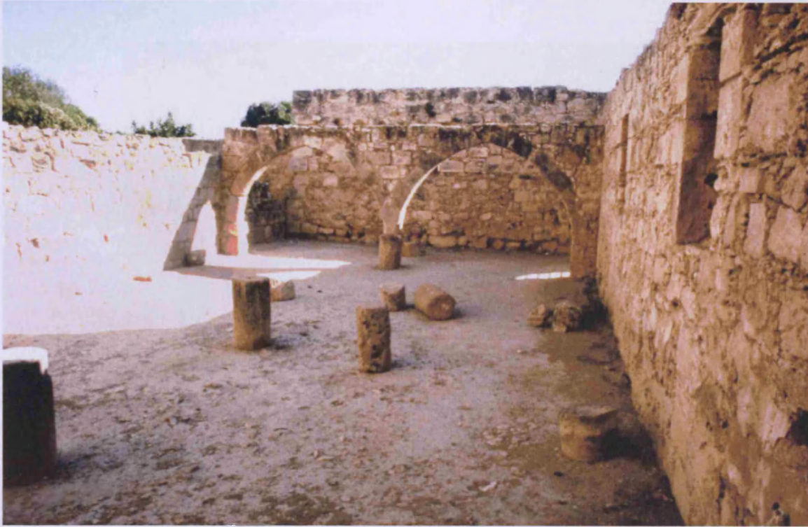
Screen formed by two pointed arches (9 on plan) in south-west corner of compound.
