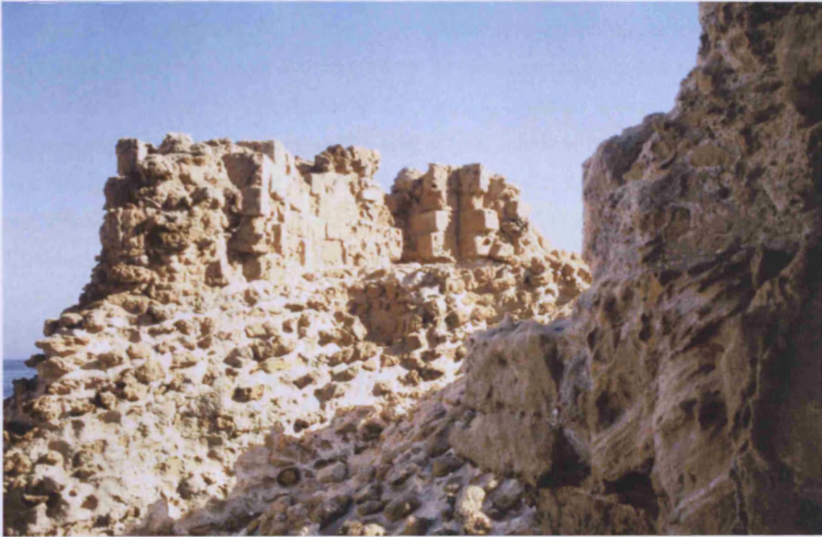
Inner walls of first floor level chamber in the ruined fort at the seaward end of the mole.
