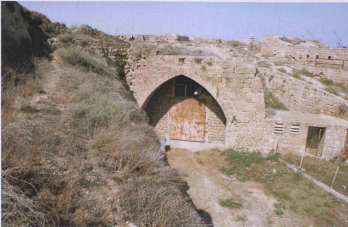
Interior of the turrus Maccelli (Genoese)/ torre del Diamante (Venetian) (15 on plan) showing its considerable pointed arched entrance.
