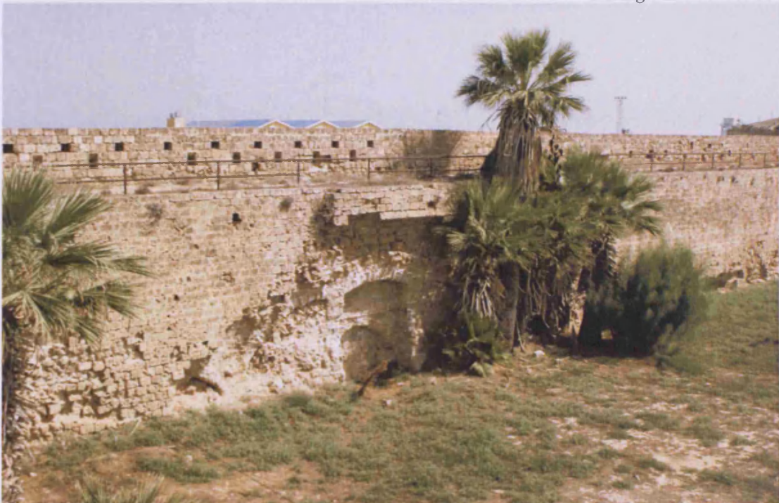
Interior of the wall between the turrus Maccelli (Genoese)/ torre del Diamante (Venetian) (15 on plan) and the turrus Morfi (Genoese)/ torre del Signoria (Venetian) (16 on plan) showing another pair of stairs rising over at least one blocked up, arched passage leading to the sea.
