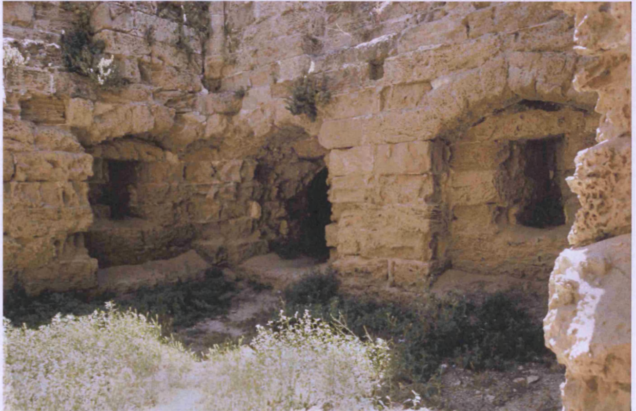
Ground level of the interior of the south-west tower (2 on plan). The archère on the outermost west side (centre in photograph) was converted to form the entrance to the tunnel to the later Venetian bastion lying beyond
