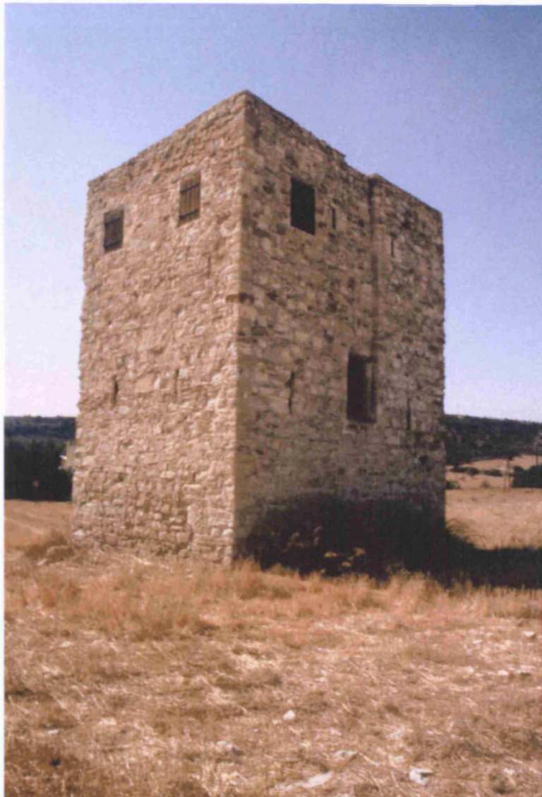
Face with supposed 'entry' at first floor level at bottom of large groove bisecting the face of the tower.
