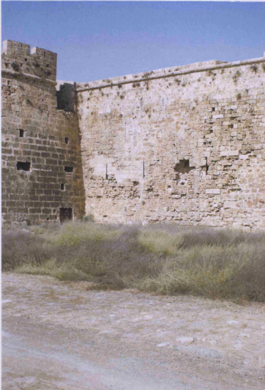
Lusignan south wall between Venetian bastions. The photograph shows one of two blocked arched passages in the wall between the Arsenal Tower and the turris Succi (Genoese)/ torre del Campo Santo (Venetian) (3 on plan). This is the western of the two. The two levels of archères are also discernible.
