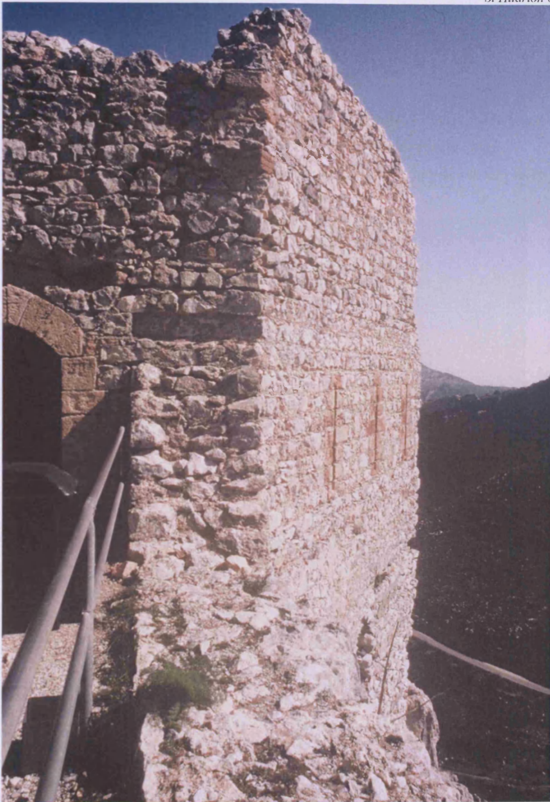
'Prince John's Tower' (32 on plan) showing its west facing entrance and the angled disposition of the rectangular tower to take advantage of the terrain. The three arrow loops on the south-west face are clearly seen.
