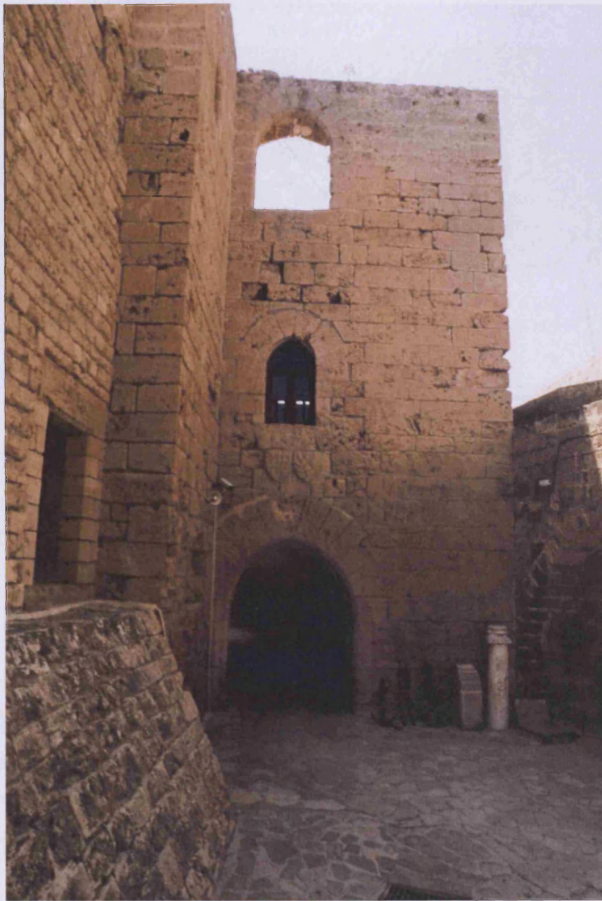
Frankish rectangular right-angled entrance (7 on plan) through the inner west curtain. The coats of arms above the entrance arch were relocated here in the early twentieth century.
