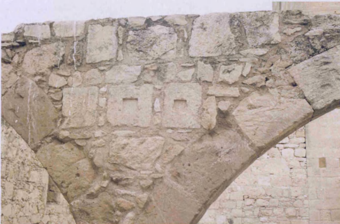
Spandrel between the two arches of the screen (9 on plan) showing two stones each with a shallow square inset.
