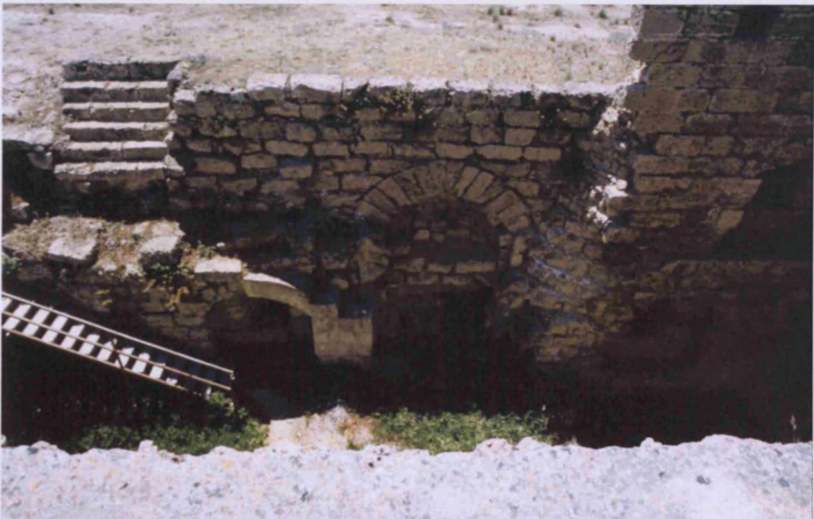
Interior of west curtain – north section, including blocked up entrance (6 on plan) with archères on either side.
