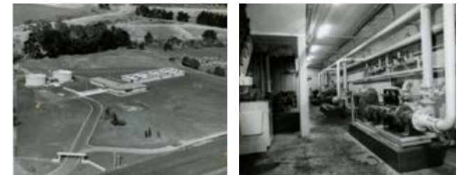
Top and bottom left photos: The pre-treatment, pumping block and operations building of the Palmerston North sewage treatment plant. Bottom right: Sludge pumping room (between pre-aeration tank and sedimentation tanks.)
