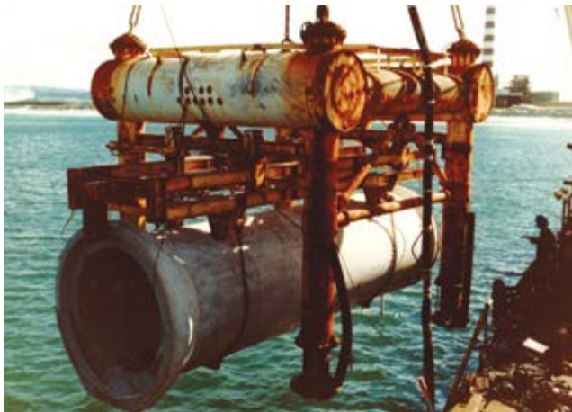
Top: February 1976, works proceeding of Marsden B with the chimney of Marsden A in the background.
