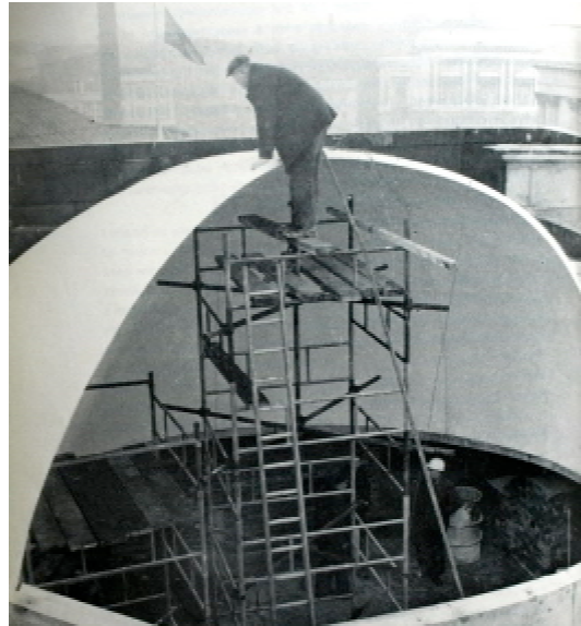
A segment of the roof of the Planetarium is slid into place. The Planetarium opened to the public in May 1970.
