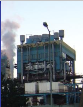
Gas/oil fired boiler 221 MW
