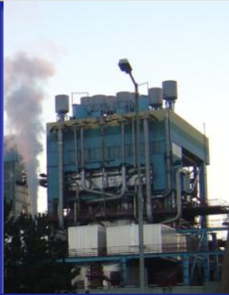
Gas/oil fired boiler 221 MW
