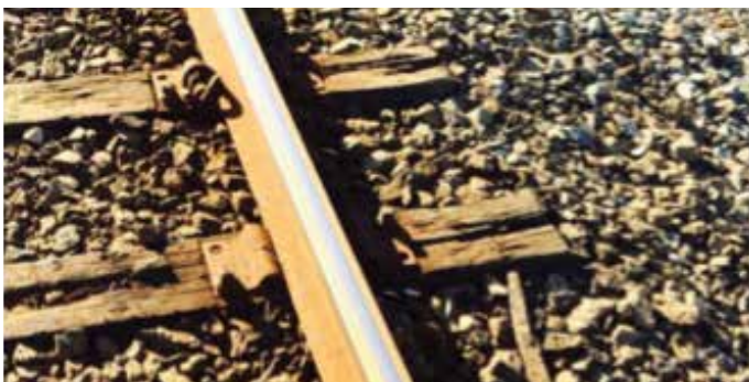
Figure 21: Example of track in poor condition
