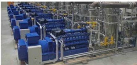
AMEC, Melbourne Water, Australia Natural Gas, Sewage Gas / 9.8 MW / 7 units
