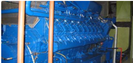
Mangga Dua Square, Indonesia Natural Gas / 14.7 MW / 8 units
