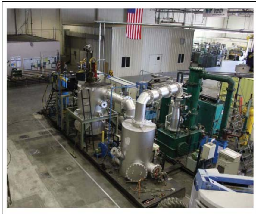
Figure 1.2-2 The PEAT System Installed at the RETC
