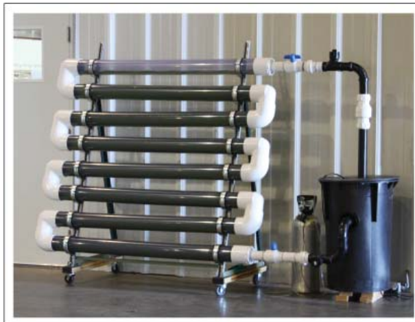
Figure 1.2-4 Ternion Bio Industries Pilot System Installed at the RETC
