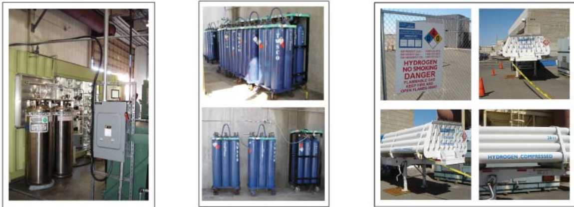
Figure 1.3-3 Examples of Gasses being Stored
