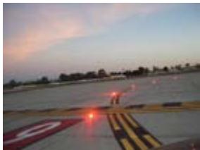
Runway Entrance Lights
