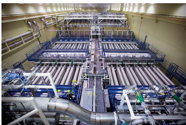
Figure 1. Top - View of the National Ignition Facility at Lawrence Livermore National Laboratory in Livermore, California. Bottom - NIF Laser Bay 2, a 96-beam bay. The yellow dots are hard hats worn by workers.
