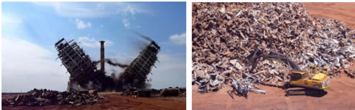
Figure 2: BHP HBI Process Plant brought down by explosives and reduced to scrap Sources: http://pilbara.me/tag/port-hedland/ & http://www.genesisattachments.com/u_boodarieironplantaustralia.asp
