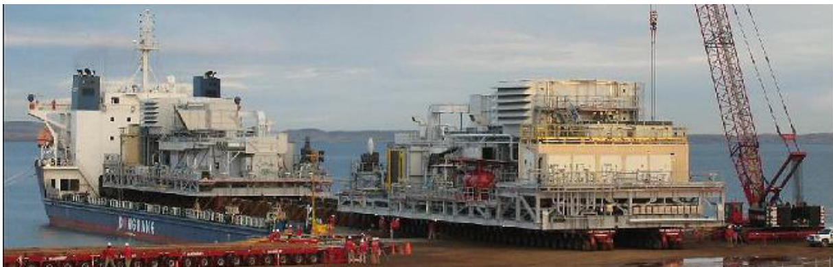
Figure 7: Pluto Process Modules being unloaded at Burrup Peninsula from special transporter ship Source: http://www.theaustralian.com.au/archive/business/woodside-petroleum-backs-off-pluto-fid-expansion-target/story-e6frq9ef-1225896105321
