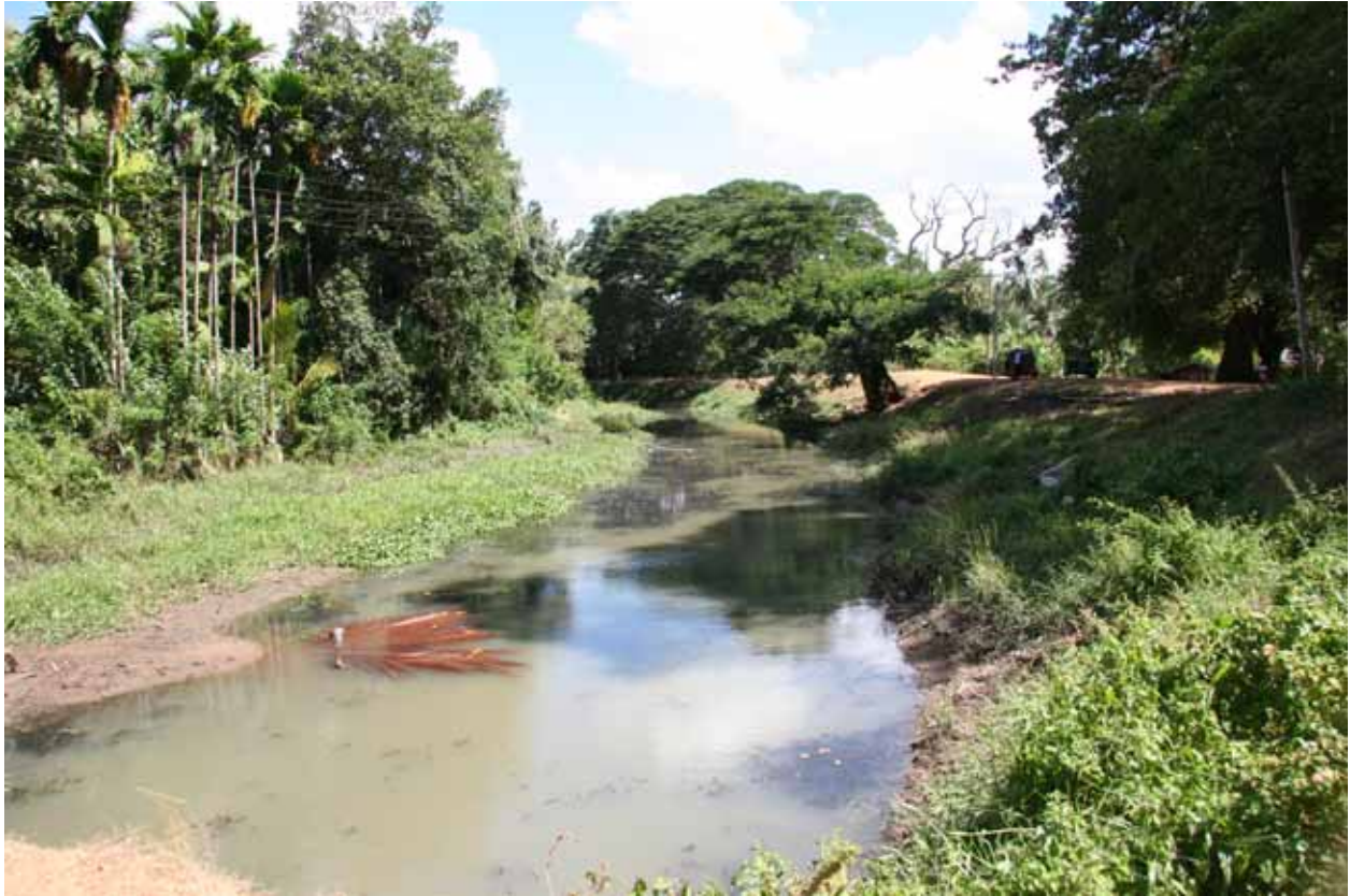
Photo 7 An ancient feeder canal that lies just below the recent replacement shown in Photo 6. Note the almost stationary flow, due to construction along the contours. The embankment is only on the lower side, enabling the canal to trap surface runoff along its way.
