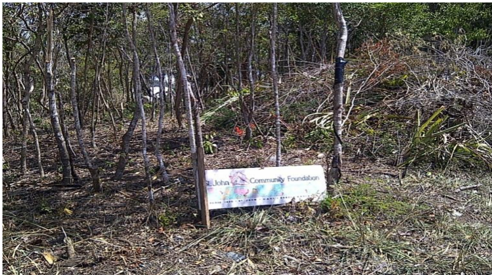
First stage of clearing a path on the St. John Community Foundation site
