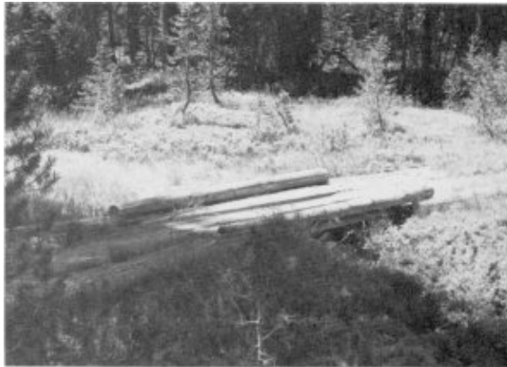
Illustration 164. Single stringer log and plank foot/horse bridge on trail between Chain Lakes and Chiquito Pass. Photos by Robert C. Pavlik, 1985.
