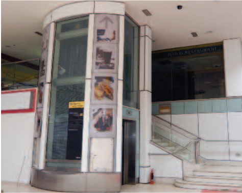
Two Storey Lift Passenger Elevator
