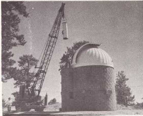
FIGURE 15. Installation of tube of 16-inch Cassegrain in J. P.L. Table Mountain Observatory. Summer of 1962.
